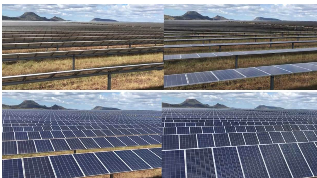
Plate 2-4: East-West Single Axis Tracker System, Finished Array
