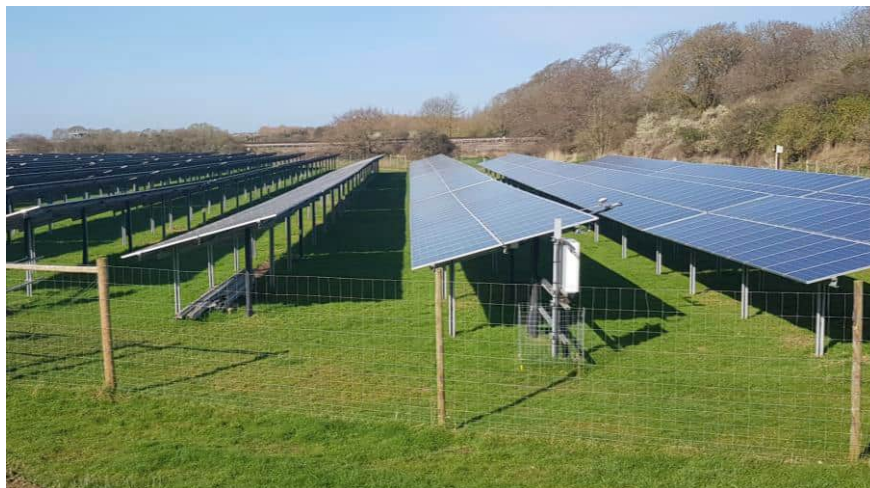
Plate 2-2: South-facing Fixed Tilt Modules, Finished Array
