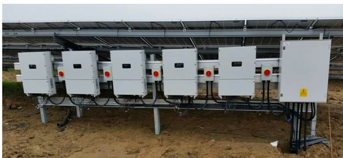
Plate 2-5: Typical String Inverter Installed under PV Modules
