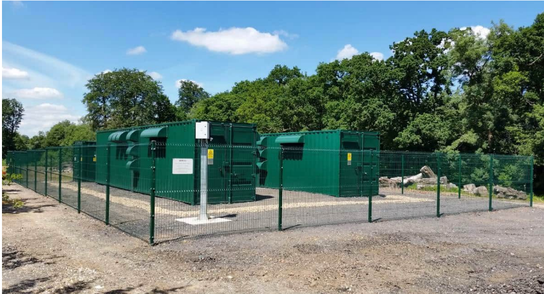
Plate 2-6: Typical Central Inverter and Combined Substation
